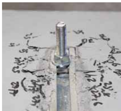
Concrete spalling on surface under tension loading
