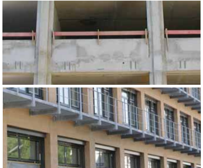
Escape walkway with vertically installed HZA Channels
