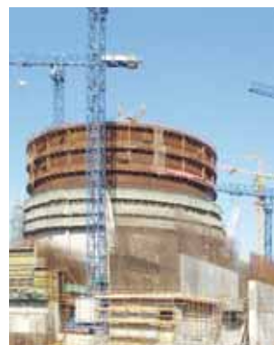
Nuclear power plant, Dalian
