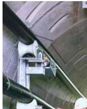
BEWAG HV utility tunnel, Berlin
